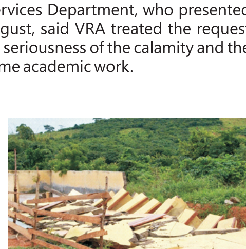
The School's collapsed KVIP
